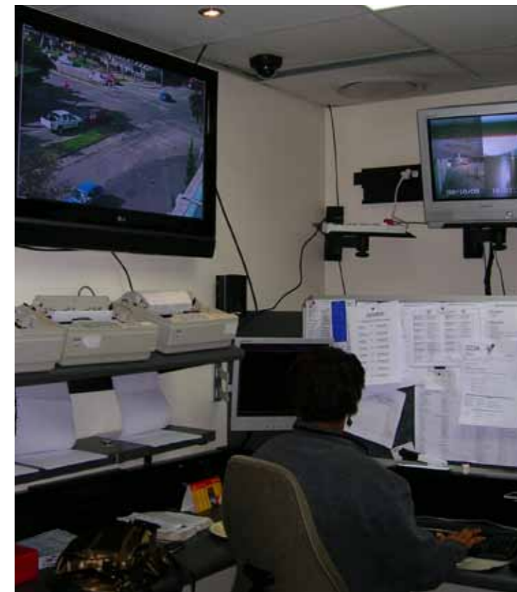
The inside of the Hi-Tec control room: a security camera on the corner of the road of Prince Alfred and Somerset Street has recently been installed.
